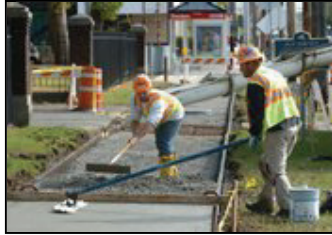
Work crews from Callanan Industries build sidewalks in Schenectady in 2010. Dolomite is a division of Callanan.
